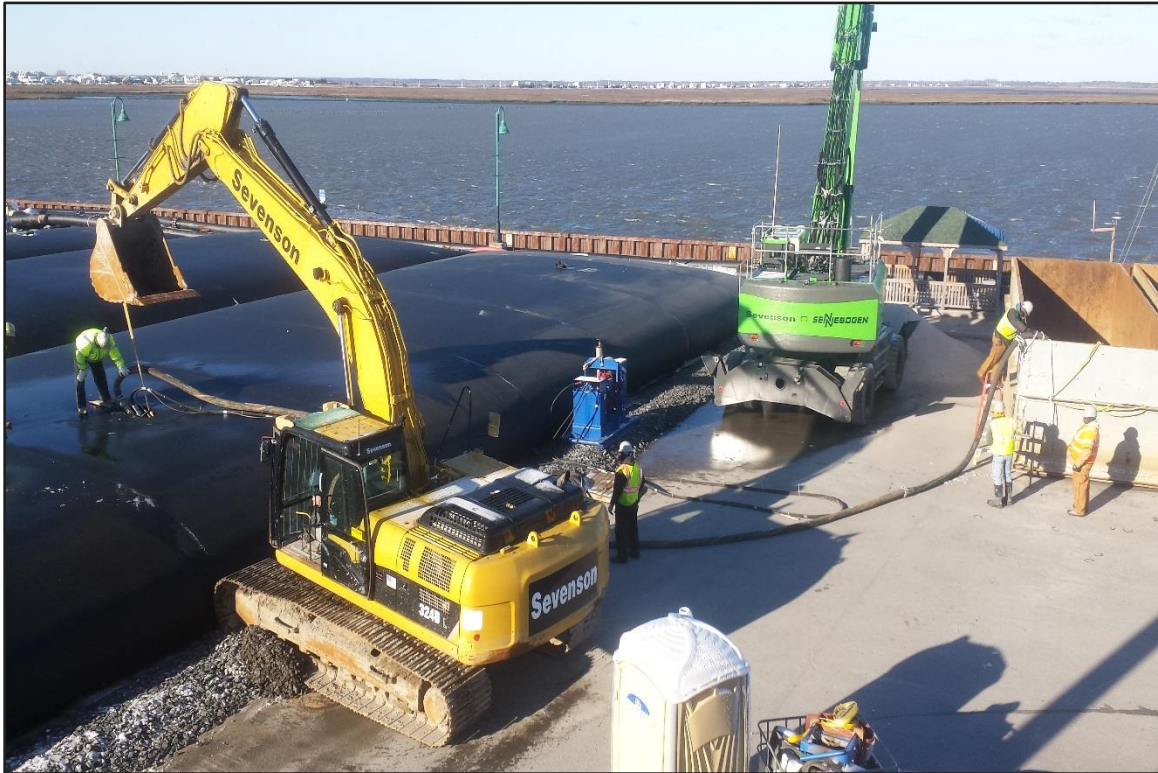
Photograph 1: De-watering Area – Pumping dredge material from geobag to mixing box. (Looking west)
