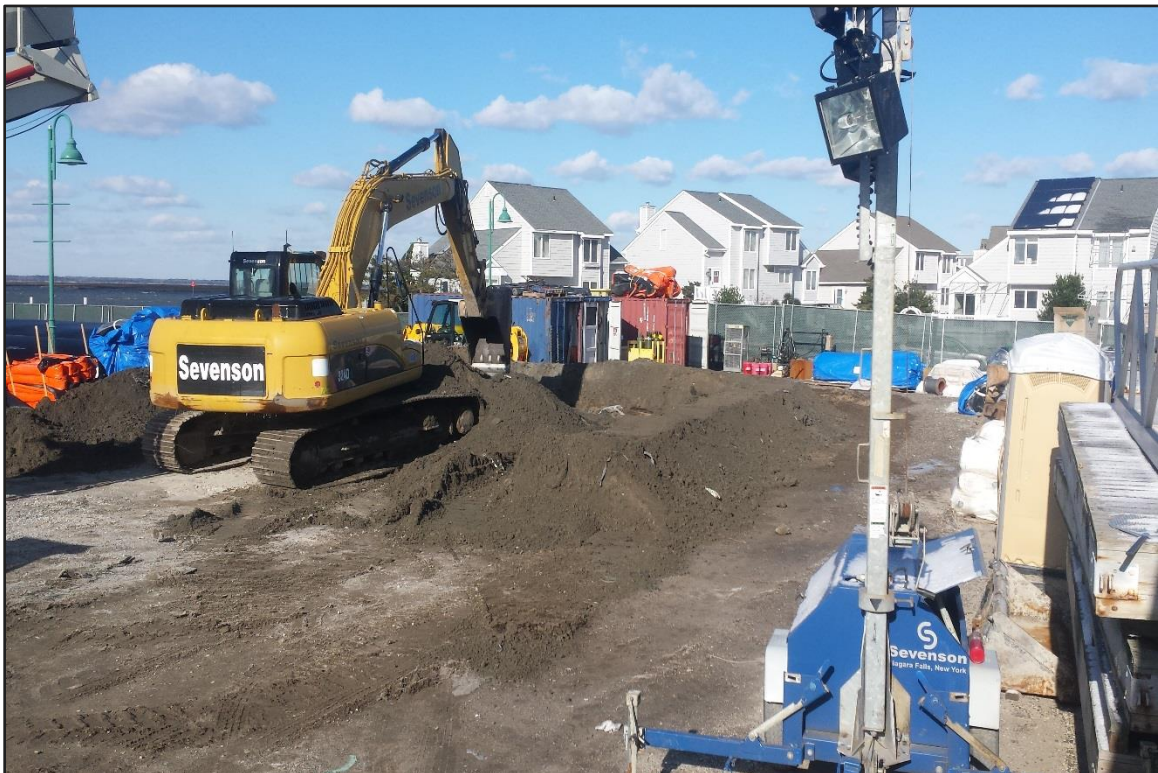
Photograph 16: De-watering Area – Creating a pit for de-watering of blended dredge material. (Looking northwest)
