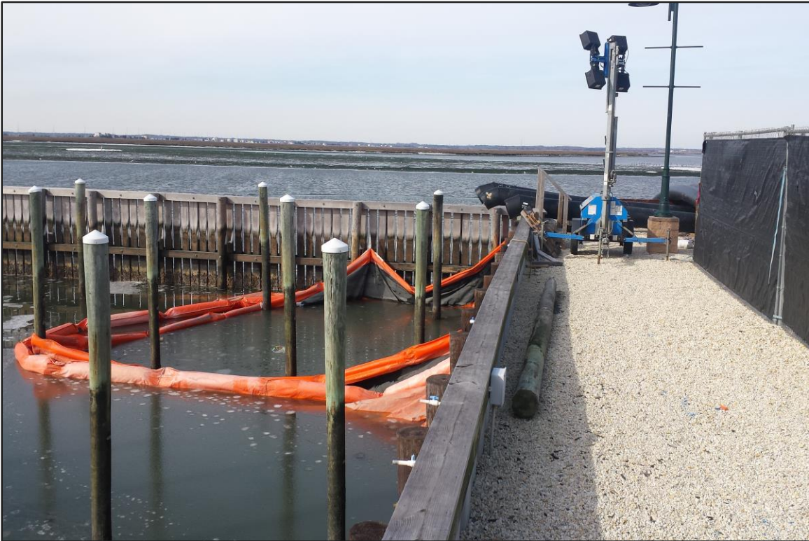
Photograph 7: De-watering area – Discharge pipes on standby. (Looking west)
