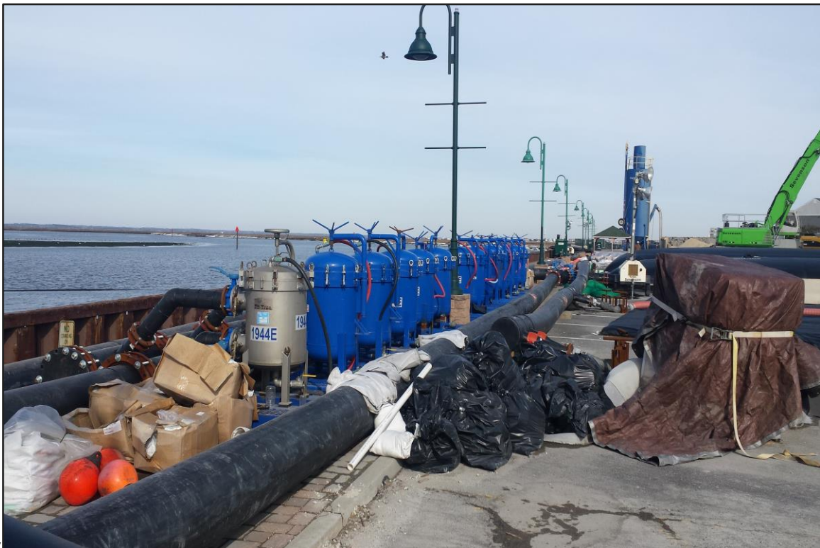
Photograph 8: De-watering area – Filtration system on standby. (Looking northwest)
