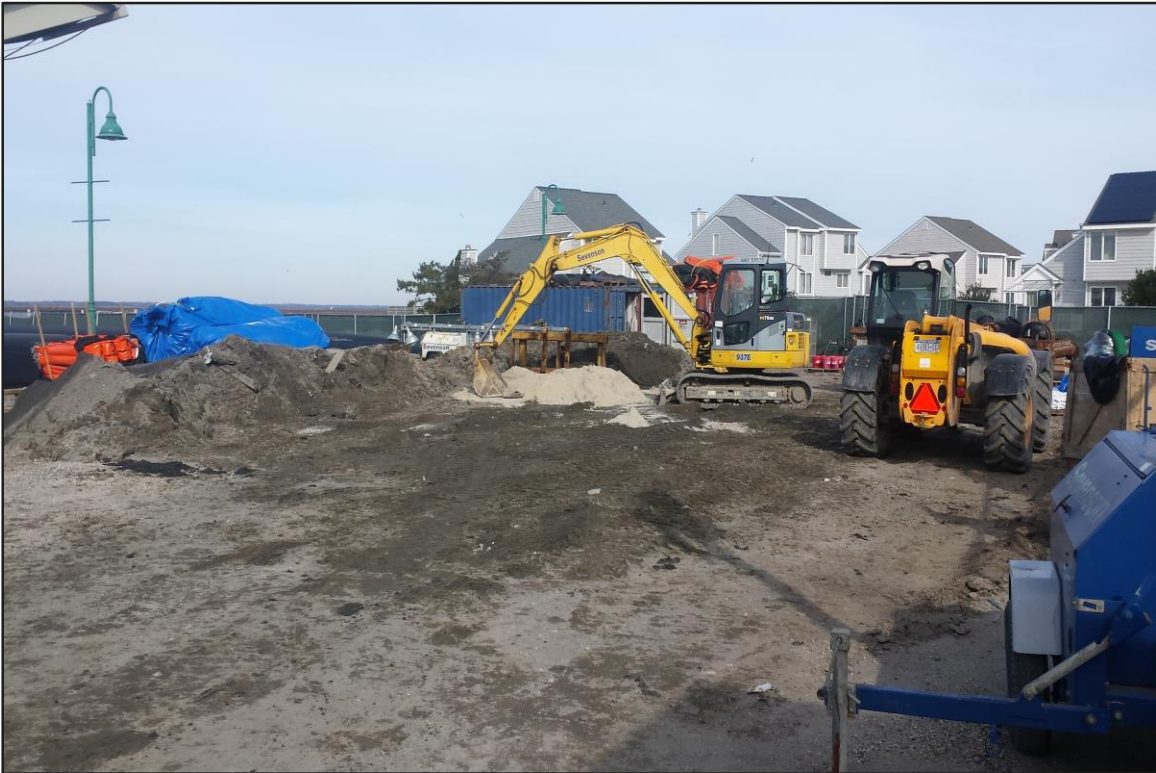
Photograph 1: De-watering area – Equipment loading sand into bags to block boat ramp. (Looking northwest)
