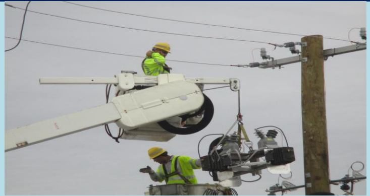
2 Atlantic City Electric lifting equipment to install on the new electrical pole.
