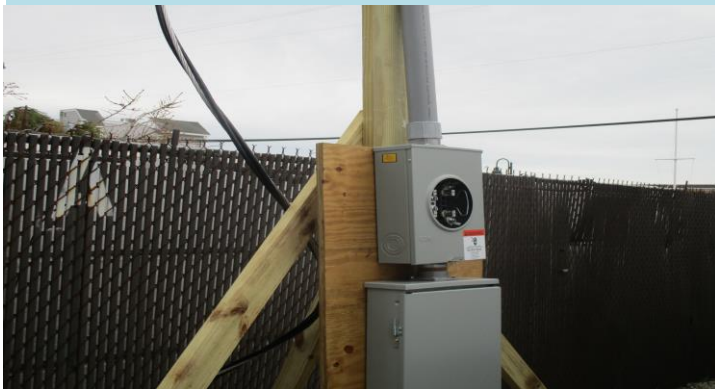
3 Meter installed for the electrical drop for the office trailers
